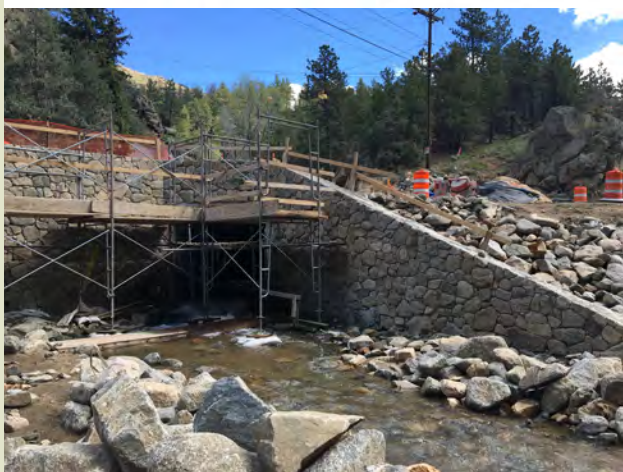
Work on Salina Junction has been in full swing. The project is still in the construction phase, as can be seen in the map to the right.
