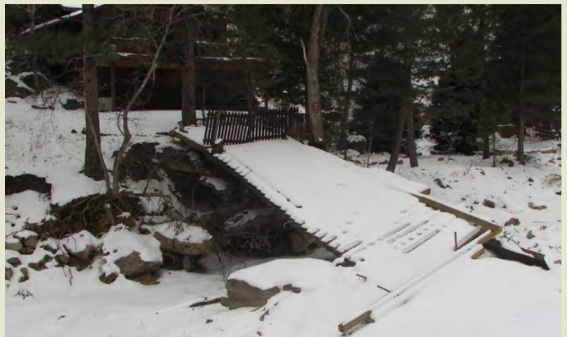
A photo of the destroyed bridge in the first winter after the 2013 Flood.
