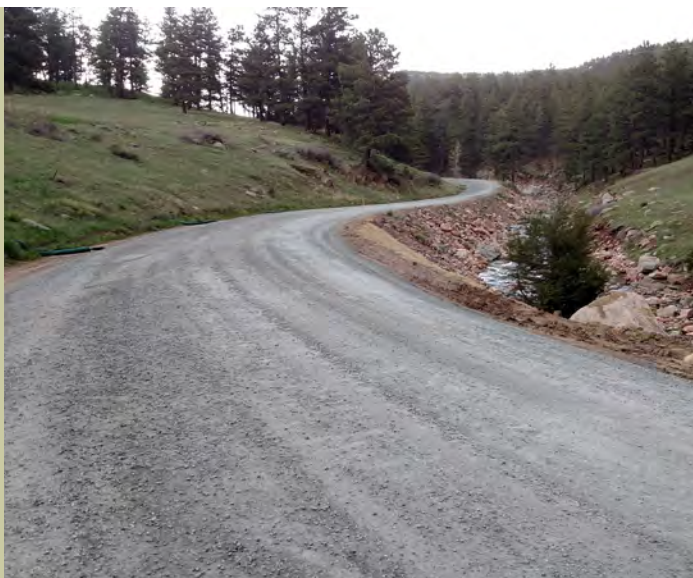
Geer Canyon Drive now has a completed road and a new completed set of culverts as of this spring.
